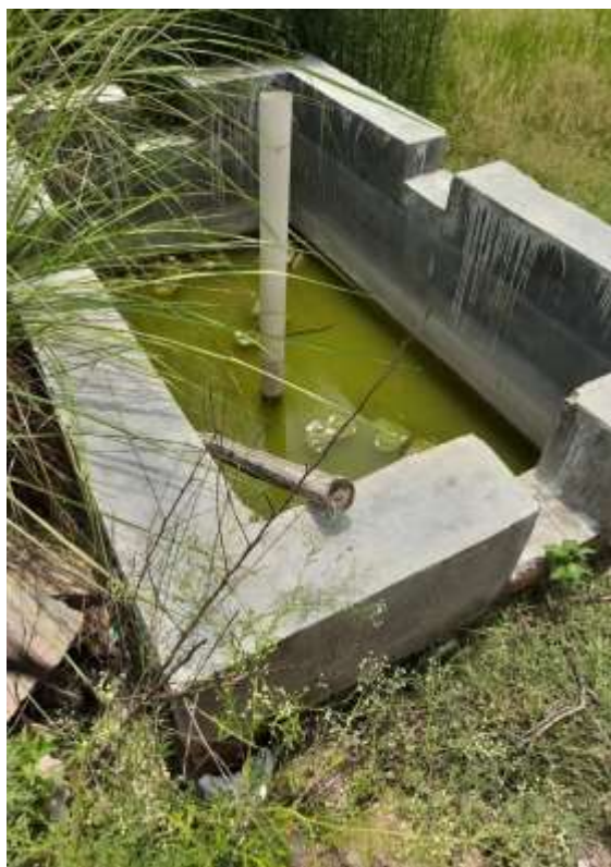
Fig. 2.4 Rain water harvesting system I located in side lawn
